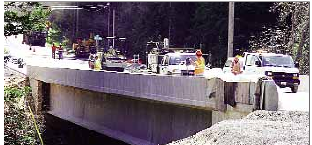
Vaughn Bay Bridge Construction 3-18-10. By March paving had begun on the bridge.
