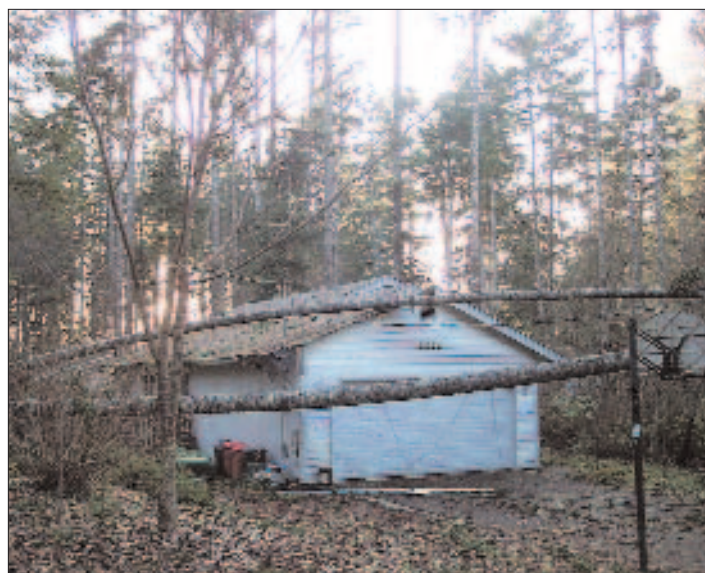
A home in Lake Minterwood sustained damage from trees that fell on the roof. Photo by Kristen Pierce
