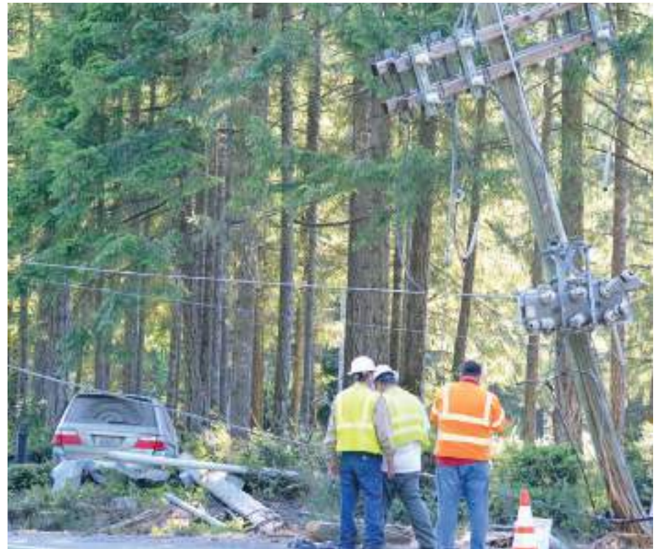
A van drove into a transformer and power pole at the three-way intersection of Key Peninsula Highway North, Lackey Road and Jackson Lake Road on the afternoon of July 29. The driver was transported to a hospital. The transformer was destroyed, starting a small brush fire, and some residents south of Home reportedly lost power, internet, landline and cell phone service for up to 12 hours. Photo: Lisa Bryan, KP News
