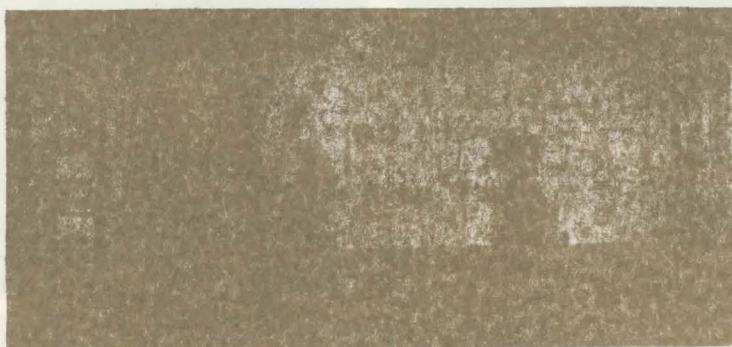
BRISTOL'S DYNAMASTER and Metagraphic instruments on this panel help monitor and control complex soybean processing operation in award-winning Chattanooga, Tennessee, plant of Central Soya Company. Entire operation is supervised from this board.
