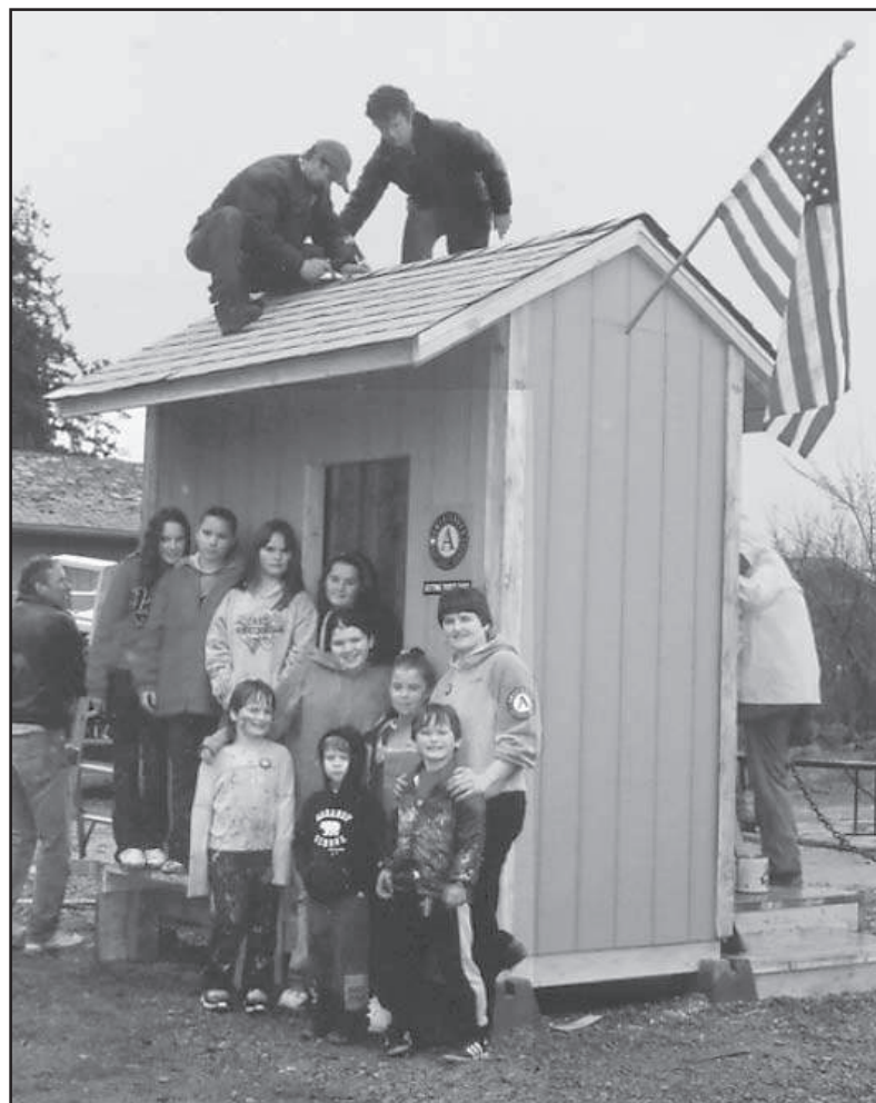
AmeriCorps-led volunteers rebuilt the school bus shelter near the Herron Island ferry landing.
