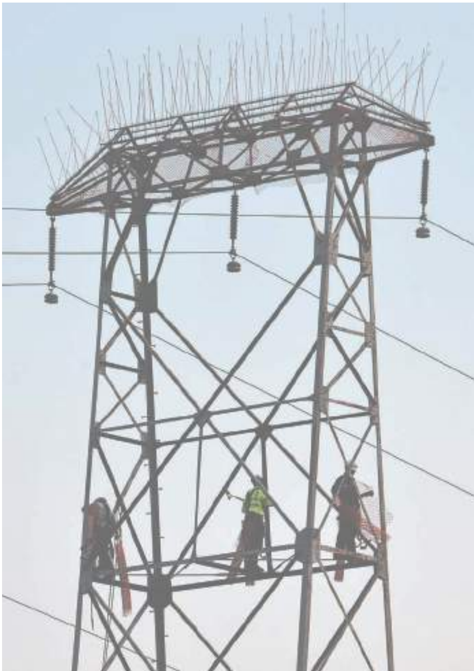
Tacoma Power workers installed bird deterrents on the towers on Purdy Spit in September in preparation for the removal of the towers later this year. Tacoma Power does not want birds living in nests when it is time to remove the towers in the future. The four existing towers, straddling Purdy Spit and in the Burley Lagoon, are over 90 years old and have exceeded their life expectancy. An additional tower will be built in the lagoon with a platform for a raptor nest. Cranes will be mounted on barges to remove the towers and avoid disrupting traffic on the Purdy Spit. There are no planned lane reductions or road closures anticipated. Construction on the new, taller single-pole towers should start in late 2017 and be completed in the summer of 2018. Photo: Don Tjossem, KP News
