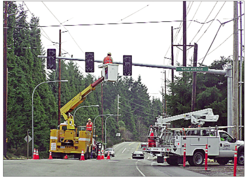
Workers were busy making the final adjustments for the new traffic light at 94th Ave. and KP Highway near Lake Kathryn Village. The light was functional by 3 p.m. Feb. 12. Photo by Mindi LaRose
