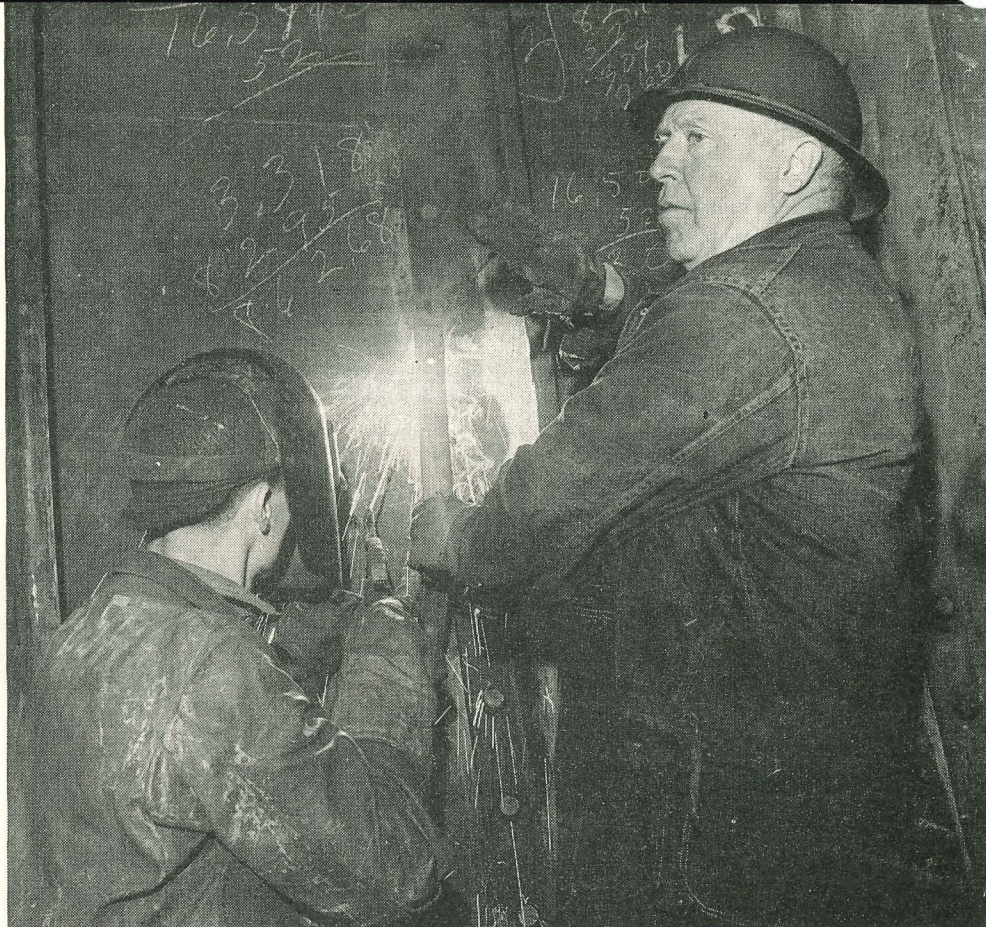
The above scene greets the eyes of Alex as he goes aboard a hull. Shipfitter Pete Griffin and Welder Julius Oster are installing wireway hangers. Pete is looking away from the job, shielding his eyes against the flash. The hanger may slip out of position. Another job to do over.
