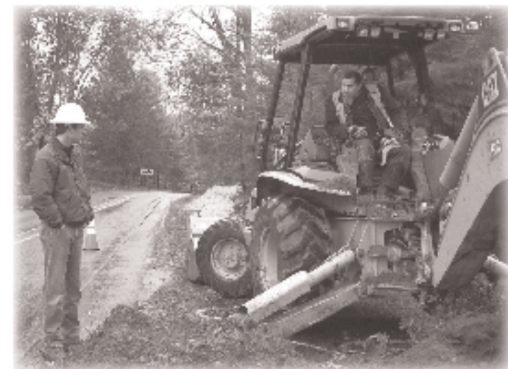
Joe Wilson, Engineering Manager, discussing the Key Center undergrounding project with ACI contractor along 92nd Ave KPN.
