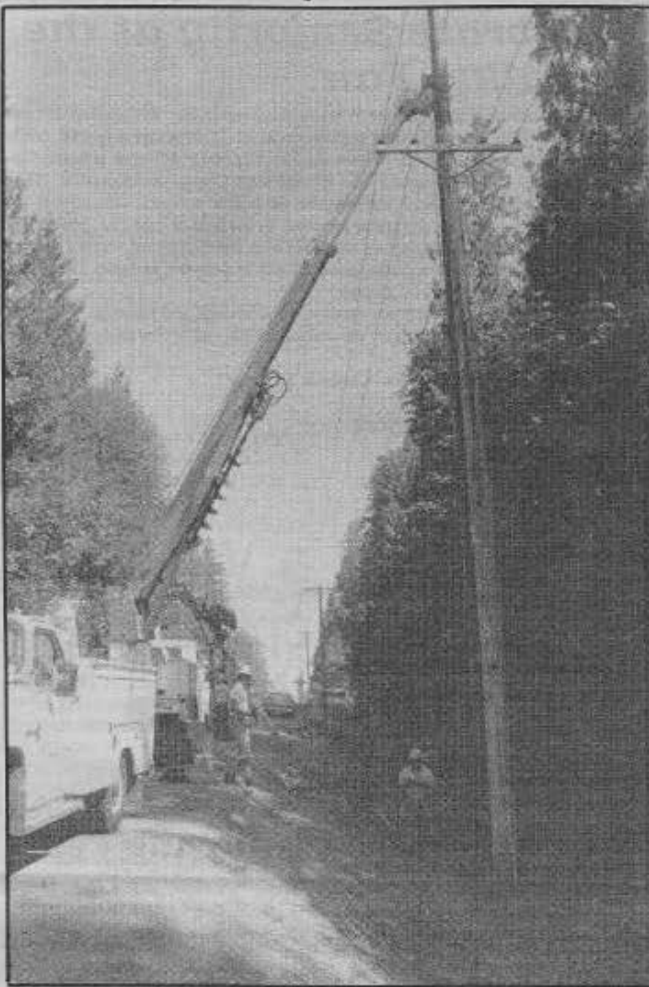
Going UP! Peninsula Light Company crew installs a new "tall" pole along Lackey Road in the central Key Peninsula area.
