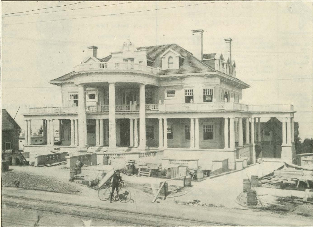
Miller & Biehn, Contractors HANDSOME STONE RESIDENCE OF WM. R. RUST, ESQ. Under Construction Russell & Babcock, Architects
