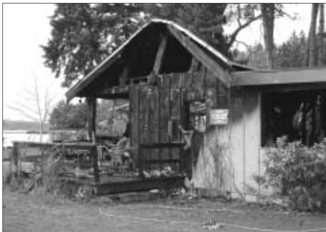
Bob McEntee's house and its contents were a total loss.
