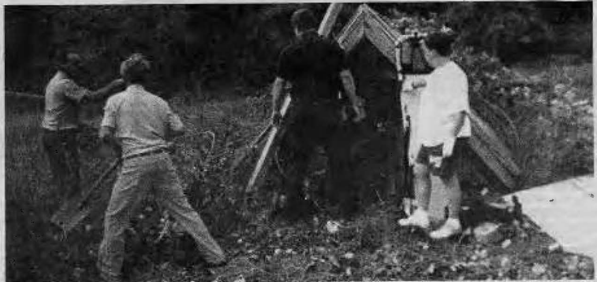
Firefighters and volunteers prepare to install a wood beam over the well
