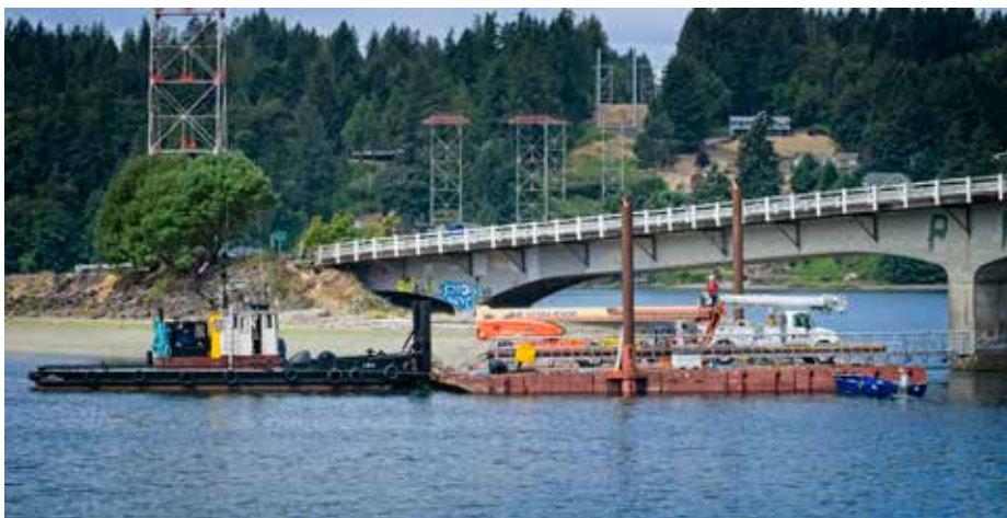
The first barge brings construction equipment to the site. Photo: Jim Bellamy
