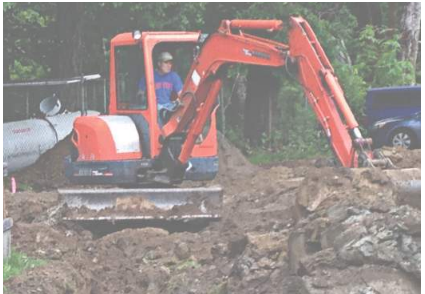
Mark Knisely digs a trench for power cables for the new emergency generator at the Key Peninsula Civic Center, which will allow it to act as an emergency shelter for residents in the event of a disaster. Photo: Ted Olinger, KP News
