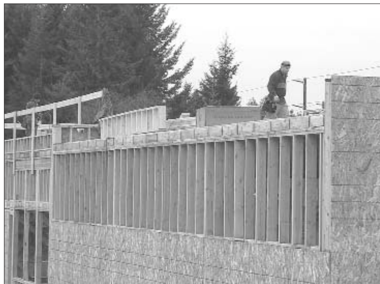
Construction of Burger King at Lake Kathryn was in full swing in December, ahead of the fast-food joint’s anticipated March opening.
