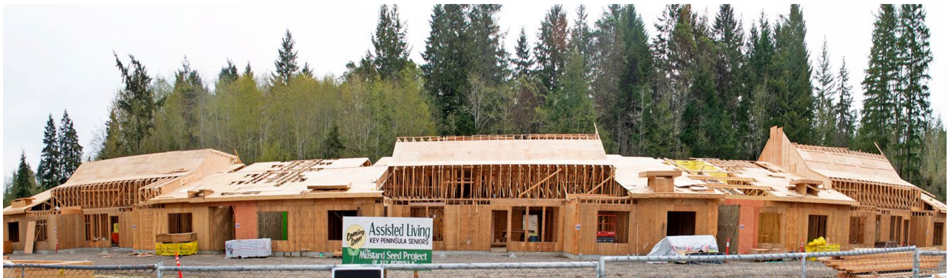
New elder homes take shape on the hill above Key Center. Ed Johnson, KP News
