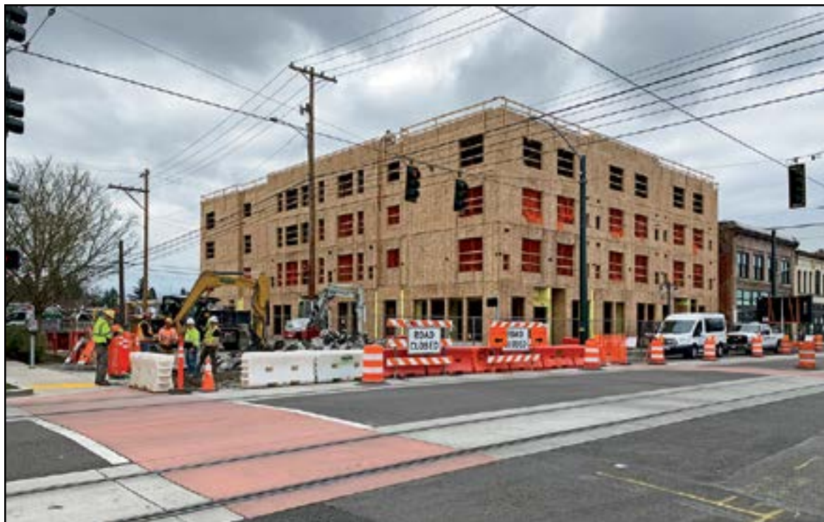
Here is a view of MLK Jr. Way and Earnest S. Brazill St. The building in construction is owned by Tacoma Housing Authority and will have commercial businesses on the first floor and affordable housing above. Mr. MAC and Sam & Terry's Barbershop will be back at this location once the building is complete.
