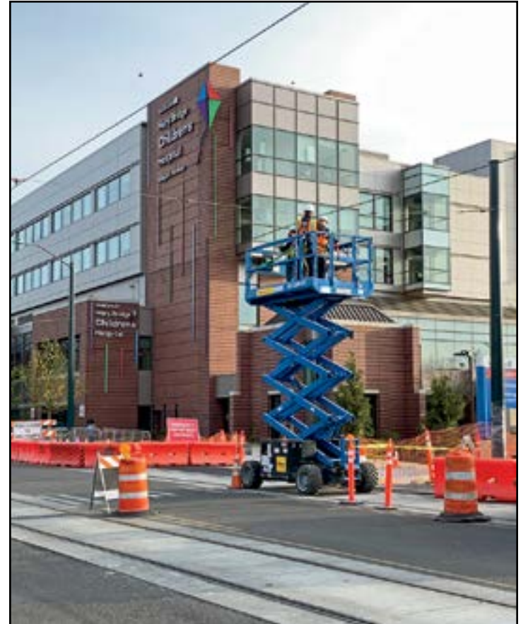
Here is photograph showing crews inspecting overhead wires near Tacoma General Hospital.
