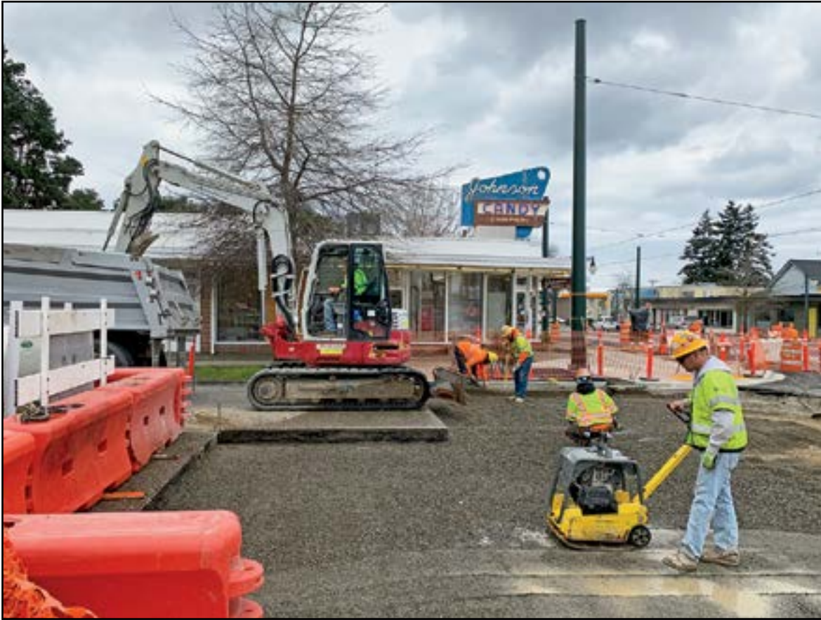
This is a great photograph showing the construction crews adding the crosswalk installation at S. 10th Street and MLK Jr. Way.
